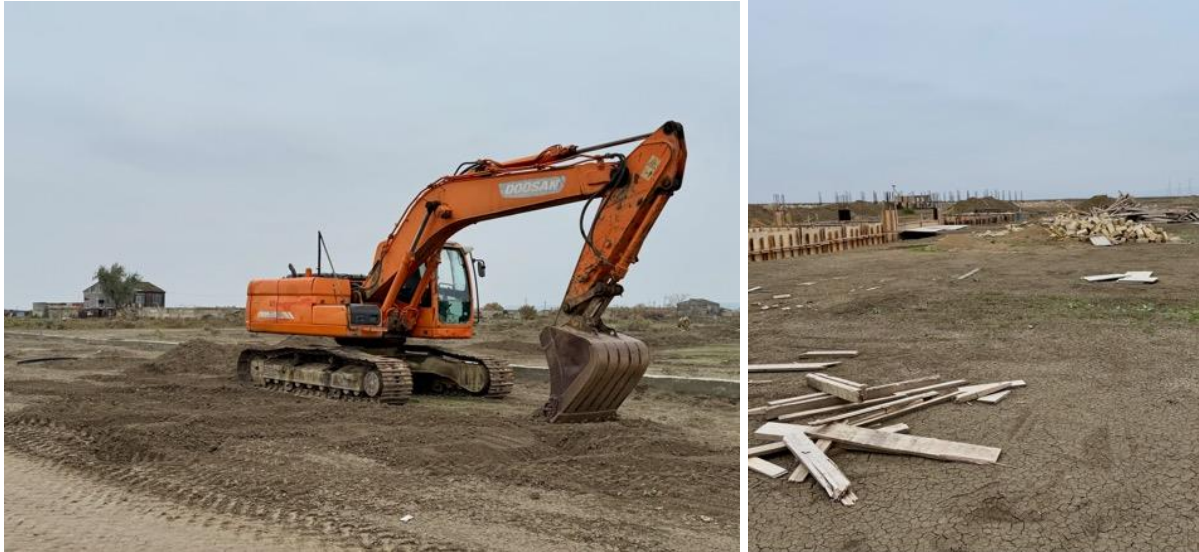
Excavator, constructed ditches and construction material at site, with nearby housing, without any fence
